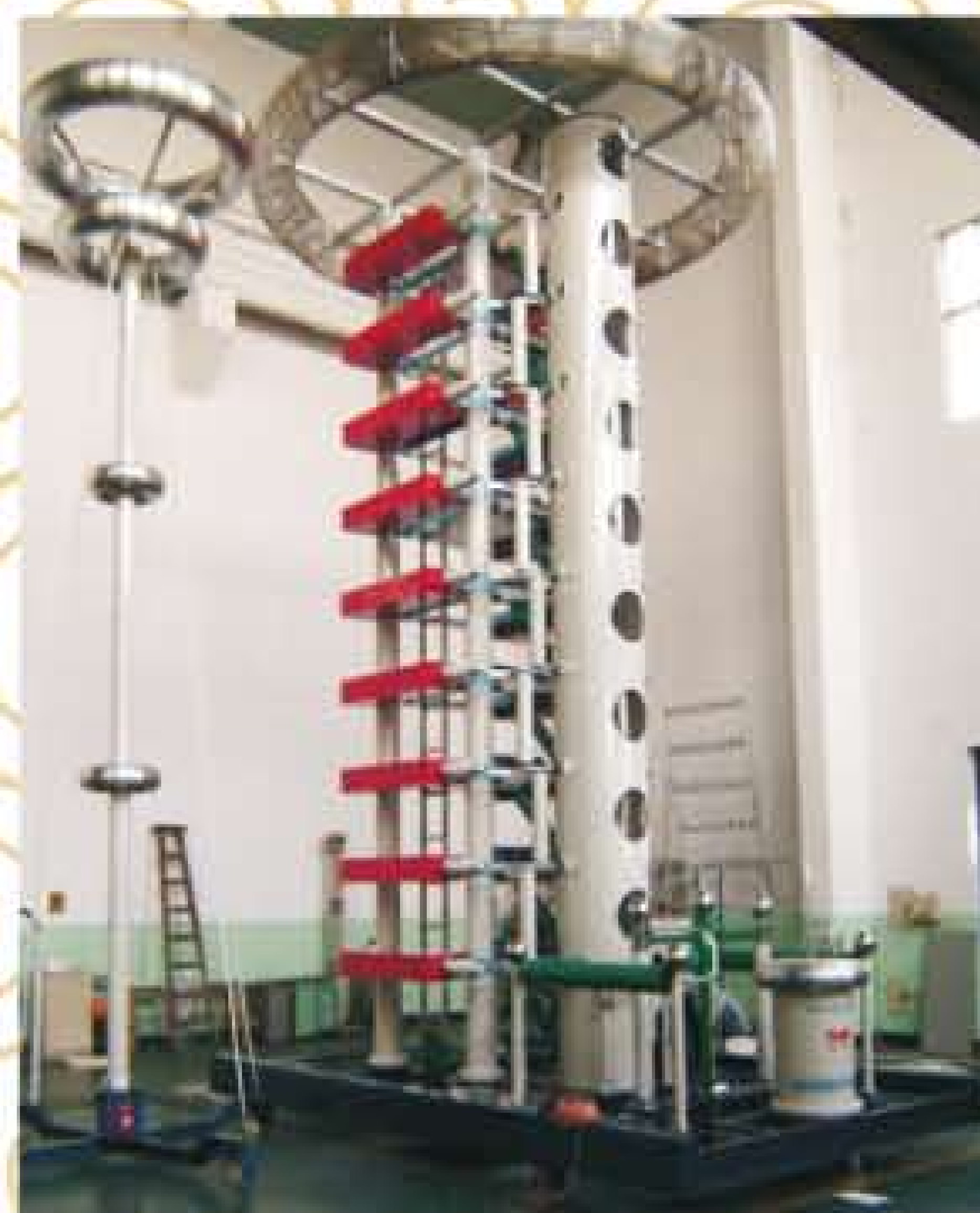
1800kV/90kJ for Transformer Manufacturer
